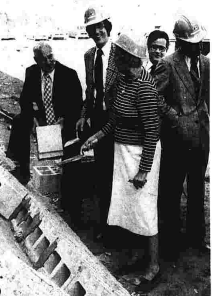
Town Manager Robert Weiss, left, and Mayor Stephen Penny help Gov. Ella Grasso to apply brick and mortar at the J.C. Penney warehouse construction site. The governor used the occasion to dramatize the state's economic vitality. Behind her are Manchester Economic Development Commission Chairman James Quigley and state Commissioner of Economic Development Edward Stockton. (Herald photo by Pinto)
